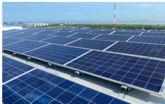
Gambar 3. Panel surya di gedung Inalum
