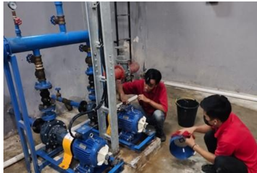
Gambar 3. Perawatan pompa transfer
