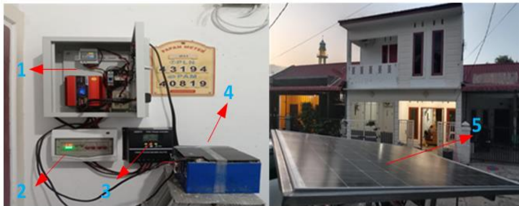
Gambar 3. Solar Home System (SHS) Off-Grid
