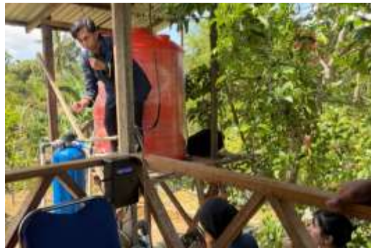
Gambar 2. Instalasi Filter Air Cerdas Berbasis IoT
